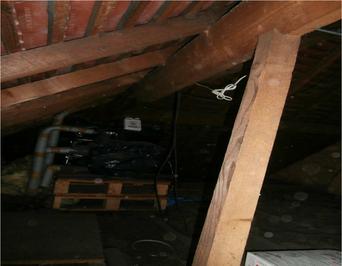
FIGURE 10 Severe twisting to the gable elevation roof purlin.
