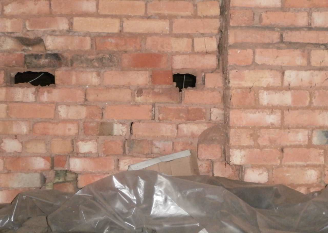
FIGURE 9 Diagonal cracking to the party wall immediately to the rear of the front chimney breast.
